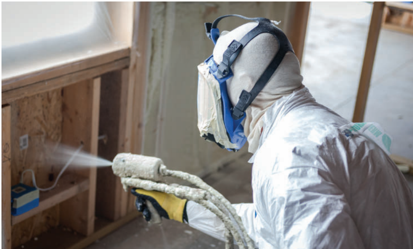
An applicator applies spray foam using Opteon™ 1100 low GWP foam blowing agent in new home installation
